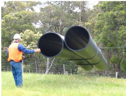
Peter McBeath, Works Supervisor, unloads the first load of 800 mm HDPE pipe
